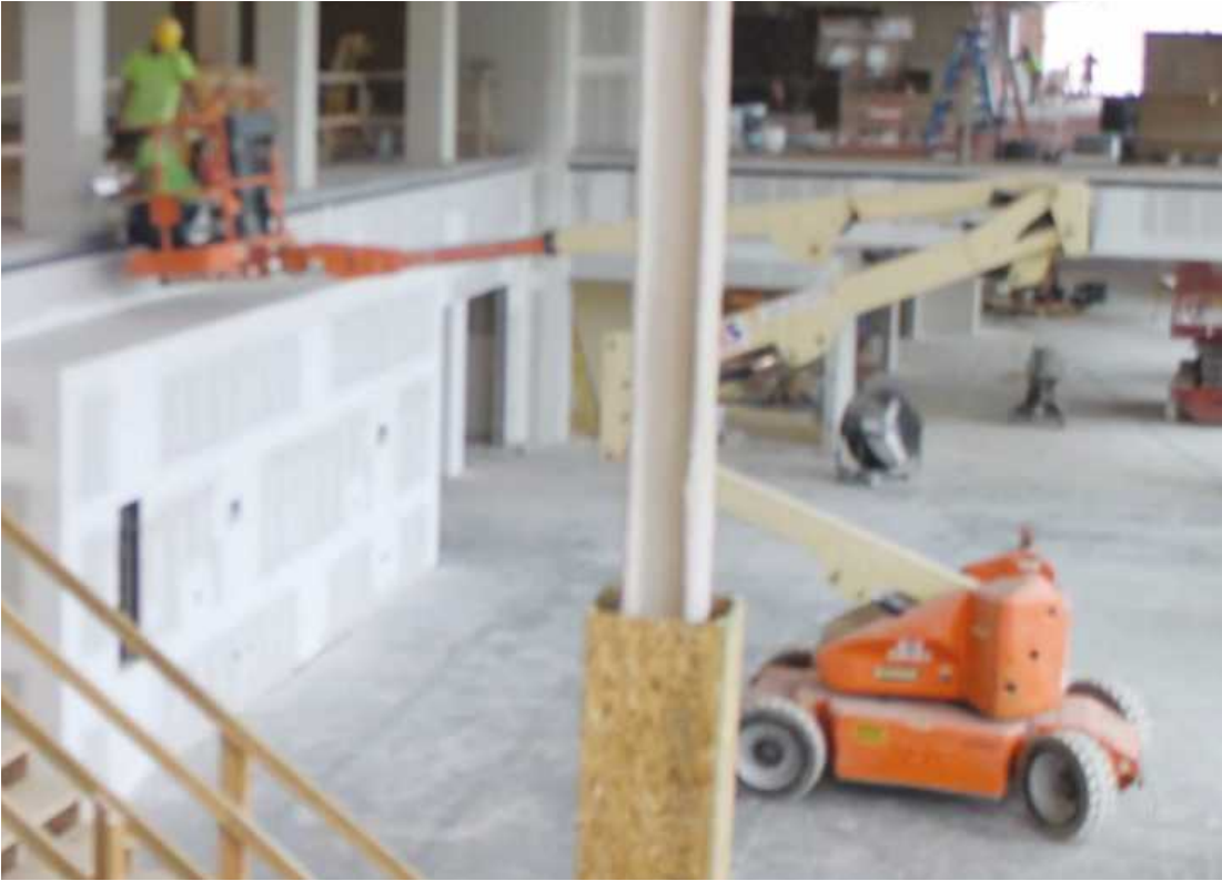
The UC has begun construction on what is to become the second Shooters location in Big Rapids.
