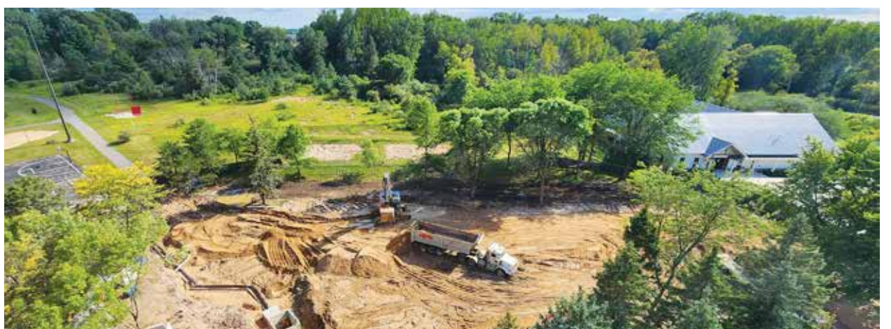
Photos by: Jordan Wilson | Multimedia Editor The demolition of Bishop hall began in early June, with site clean-up set to be complete before students return this semester.
